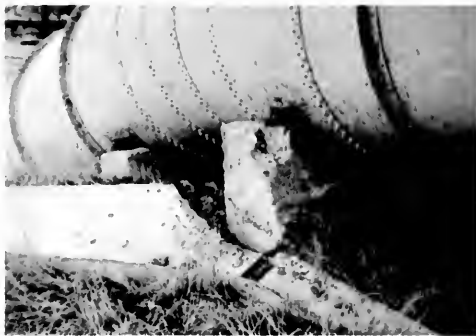
Photo 8. Part of the older Los Angeles Aqueduct pipeline just north of the Golden State Freeway where it rotated and slumped. A ground rupture in the Sunshine Ranch Member of the Saugus Formation passes beneath the broken foundation. View is south-southwest.
